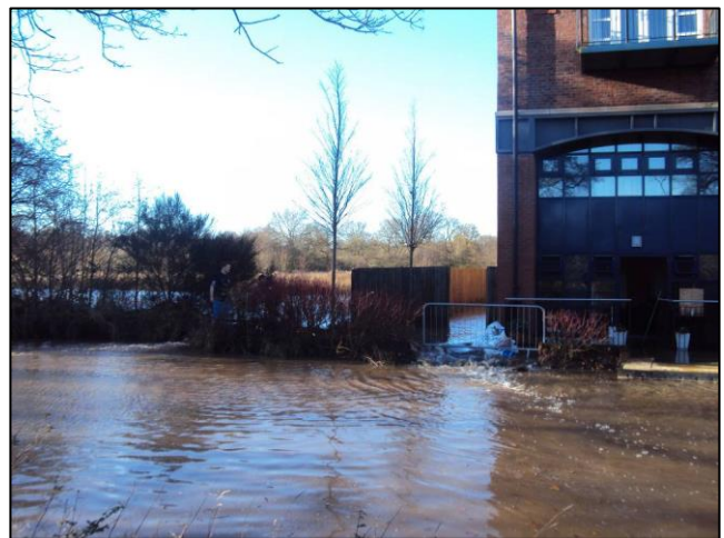
Figure 4 - Ordinary watercourse flooding in November 2012 at Dickens Heath due to a culvert inlet blockage
