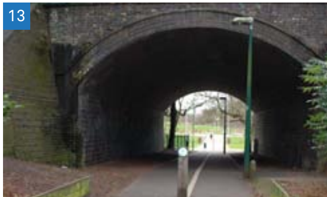
13 Railway underpass connecting Tudor Grange Park and Solihull Town Centre: the underpass can present safety concerns particularly in the evening, due to poor lighting and little overlooking.
