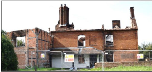
5. Castle Hills Farmhouse following fire in July 2020
